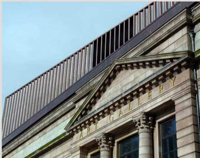
The red/brown colour of the Art Gallery roof extension reflects that of the pink Corrennie granite below.
